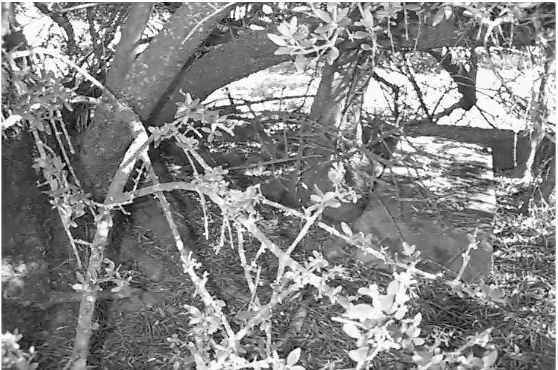
Figure 3.3. Example of a mature feral olive pushing apart the foundation of a buttress.
